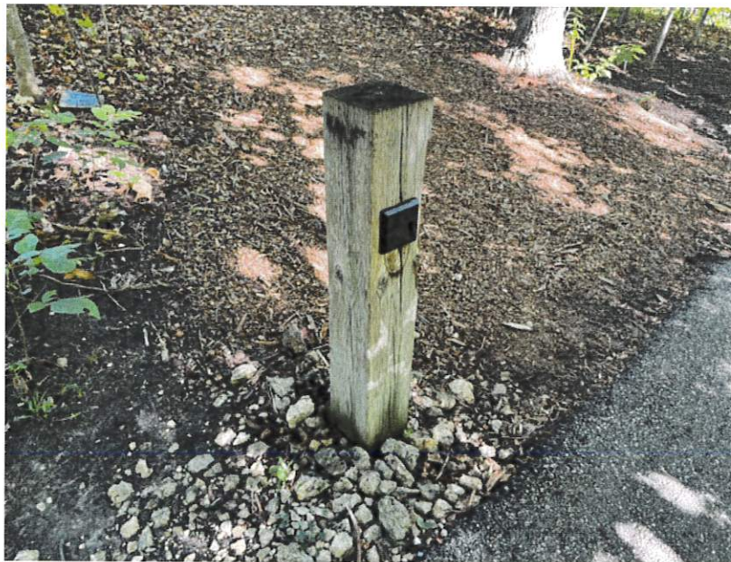
Example of path lighting at Covenant Harbor
