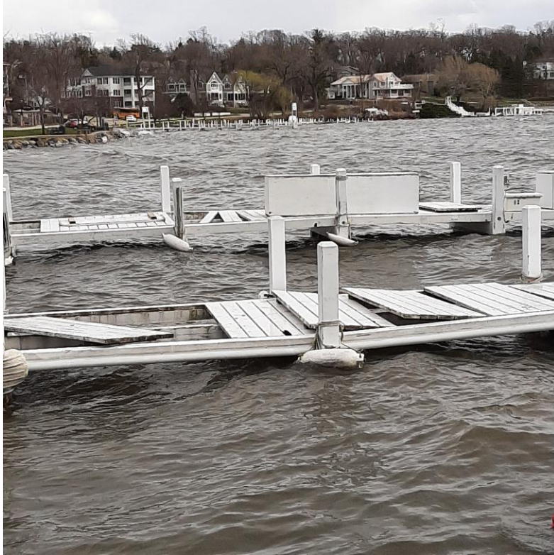
Elmer's Rental pier. Far pier out of crib; supports and stringers need replacing
