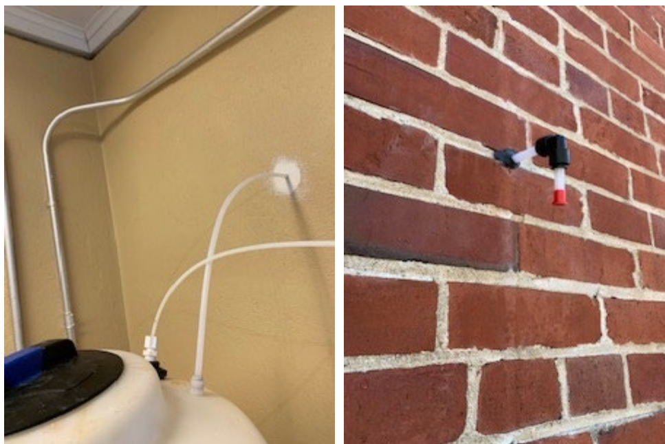
Wellhouse #2 Sodium Hypochlorite Venting
