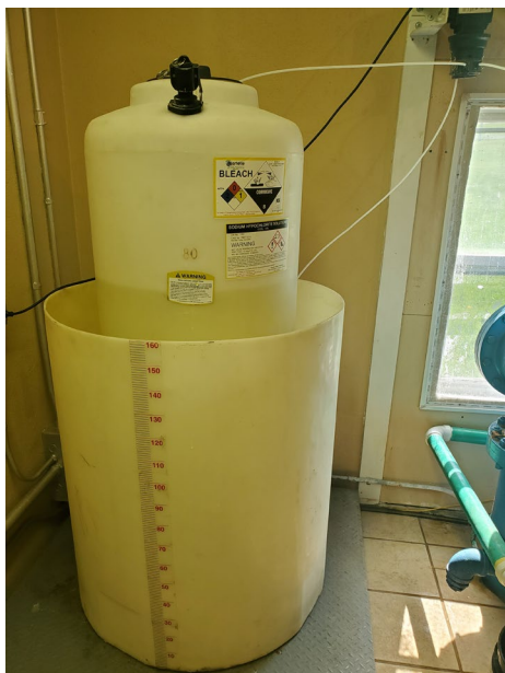
Figure 1) Hypochlorite tank lacking vent
