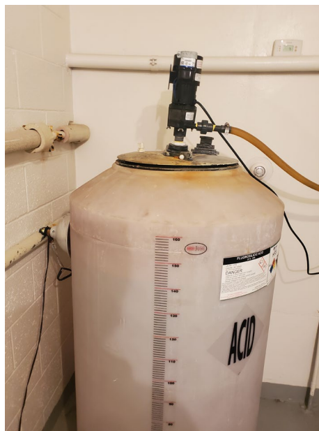
Figure 2) Fluoride tank lacking vent
