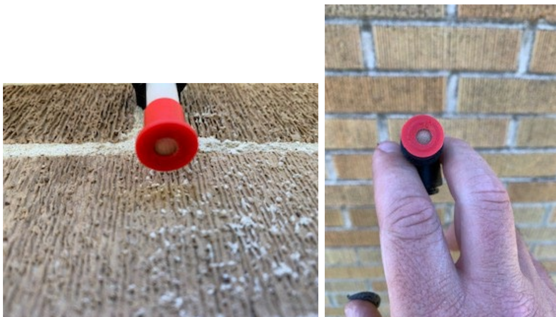
New Chemical Vents (Typical)
