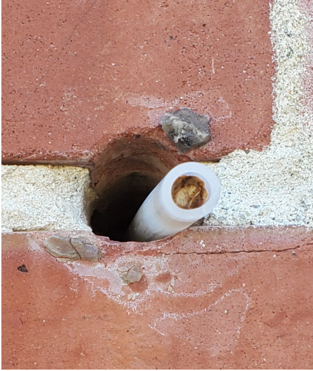
Figure 3) Vent not adequately screened or downward facing. Vent blockage evident
