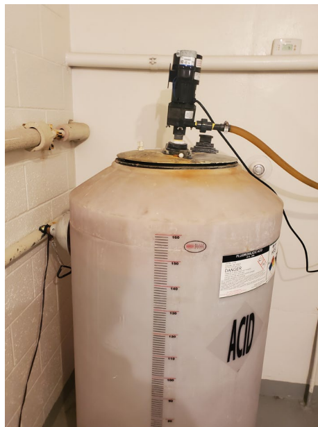
Figure 2) Fluoride tank lacking vent
