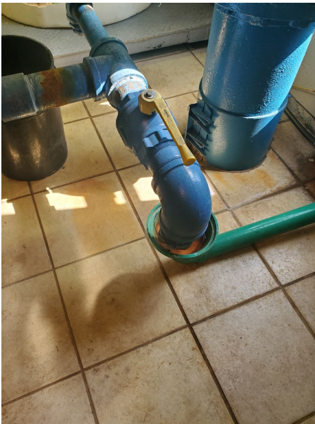
Figure 4) Well two vent not 24” above floor
