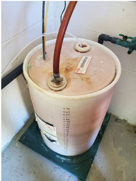
Figure 5) Fluoride day tank lacking secondary containment
