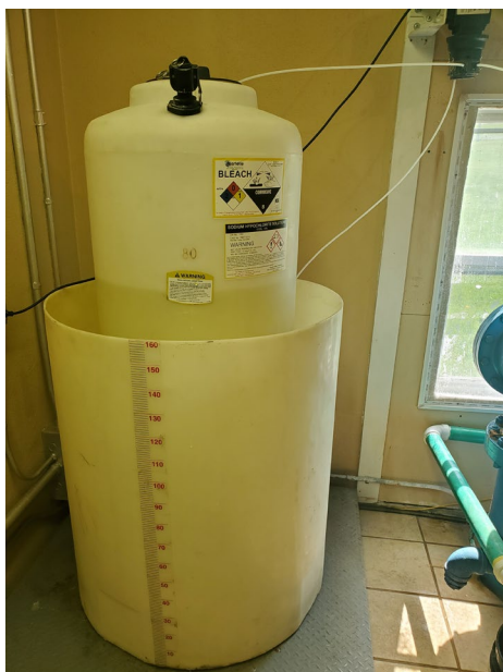
Figure 1) Hypochlorite tank lacking vent
