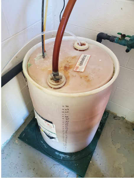
Figure 5) Fluoride day tank lacking secondary containment
