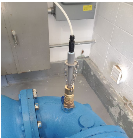
Figure 6) Chemical injection port at well 5
