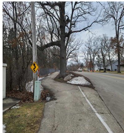
The existing path will be repaved because of deteriorating pavement conditions. Large mature trees line the existing trail and the future trail corridor.
