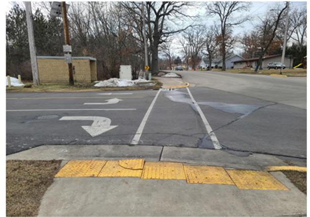
Existing curb ramps throughout the corridor are cracked and do not meet Americans with Disabilities Act (ADA) standards.
