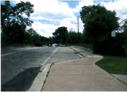
Existing bridge in need of rehabilitation.
