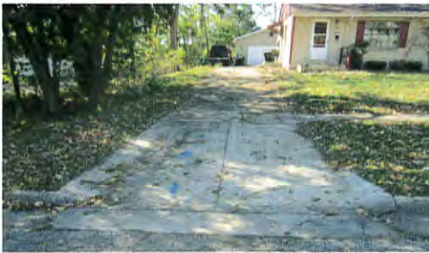
Existing deteriorated pavement and driveway apron.
