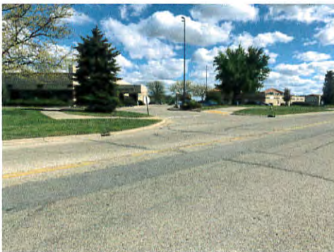
East Sheridan Springs Road existing pavement condition.
