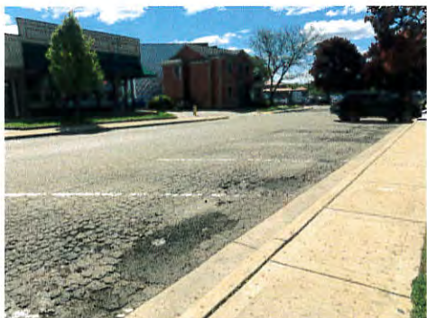
Cook Street parking lane pavement deterioration.
