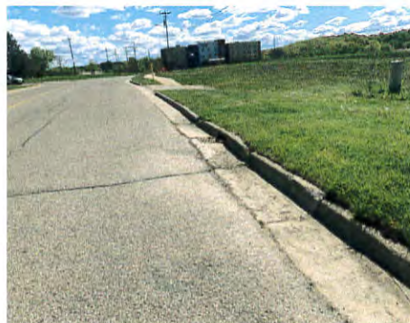
East Sheridan Springs Road curb and gutter issue at inlet.
