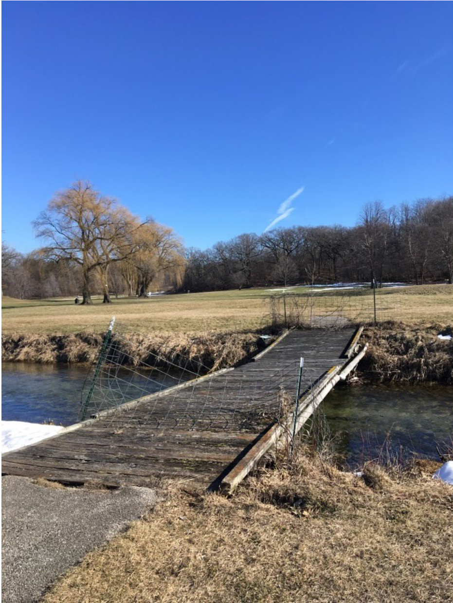
Bridge #3 (closed, unusable)
