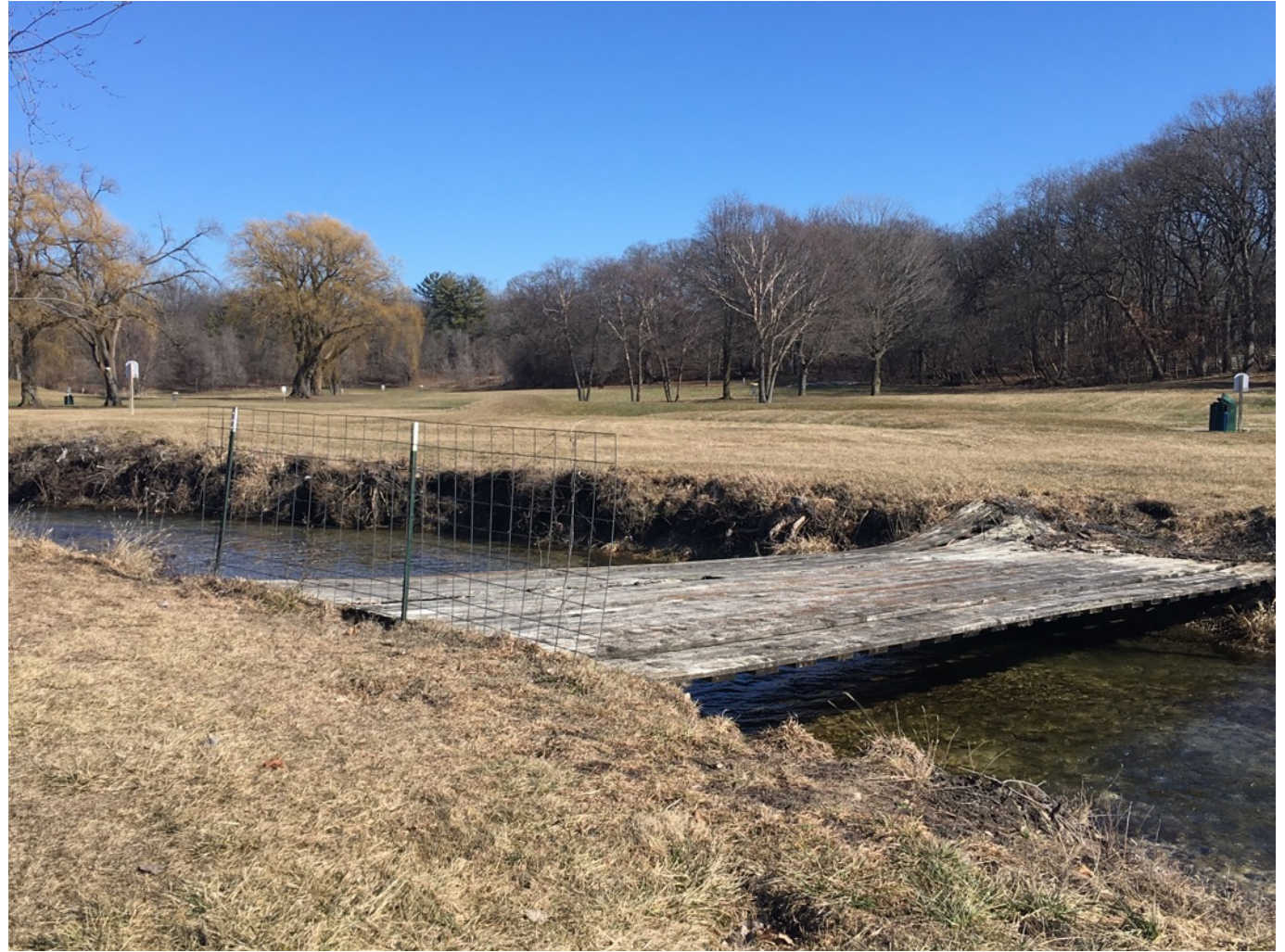
Bridge #4 (closed, unusable)
